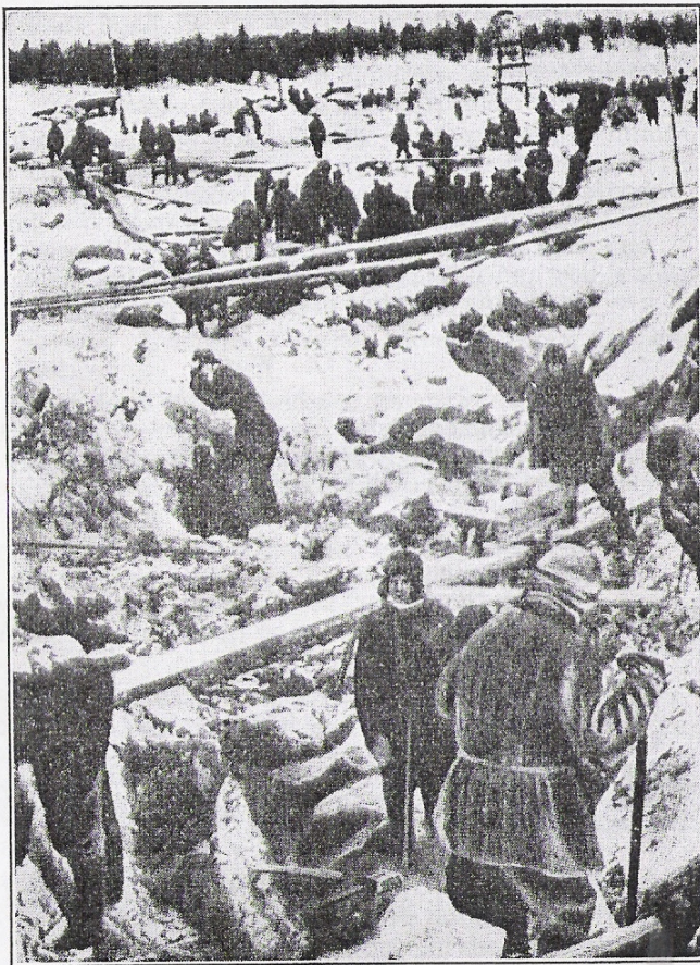
The construction of the White Sea Canal. Picks, wheelbarrows and planks—these represent the entire “technical” equipment of the compulsion workers. This picture shows that the understratum is solely composed of rock. The complete lack of machines and technical supplies alone would make the life of prisoners literally a hell.
